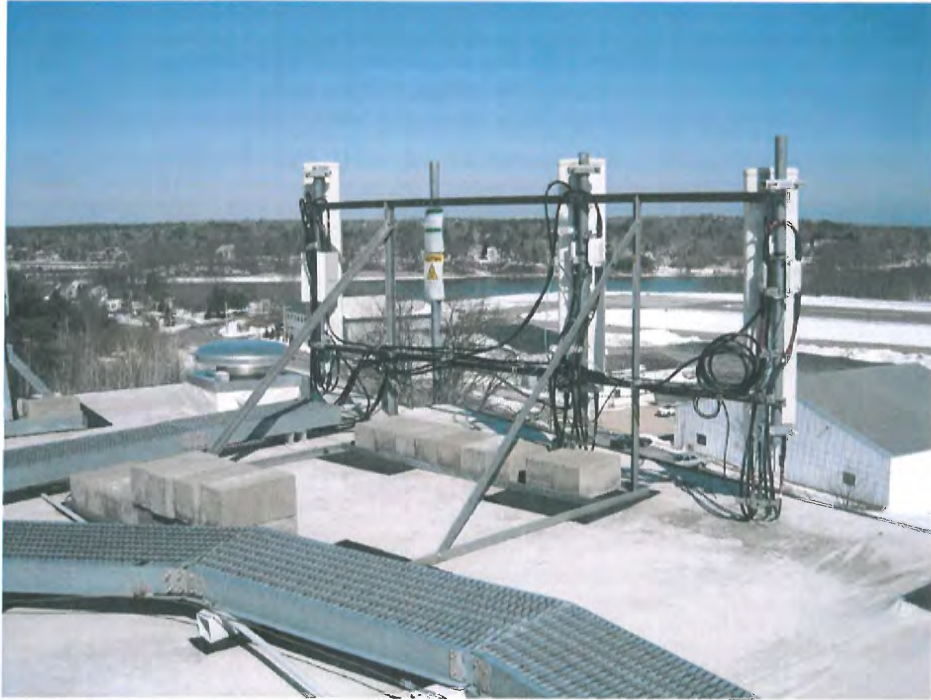
Photo 3: Sample photo illustrating the existing antennas.
